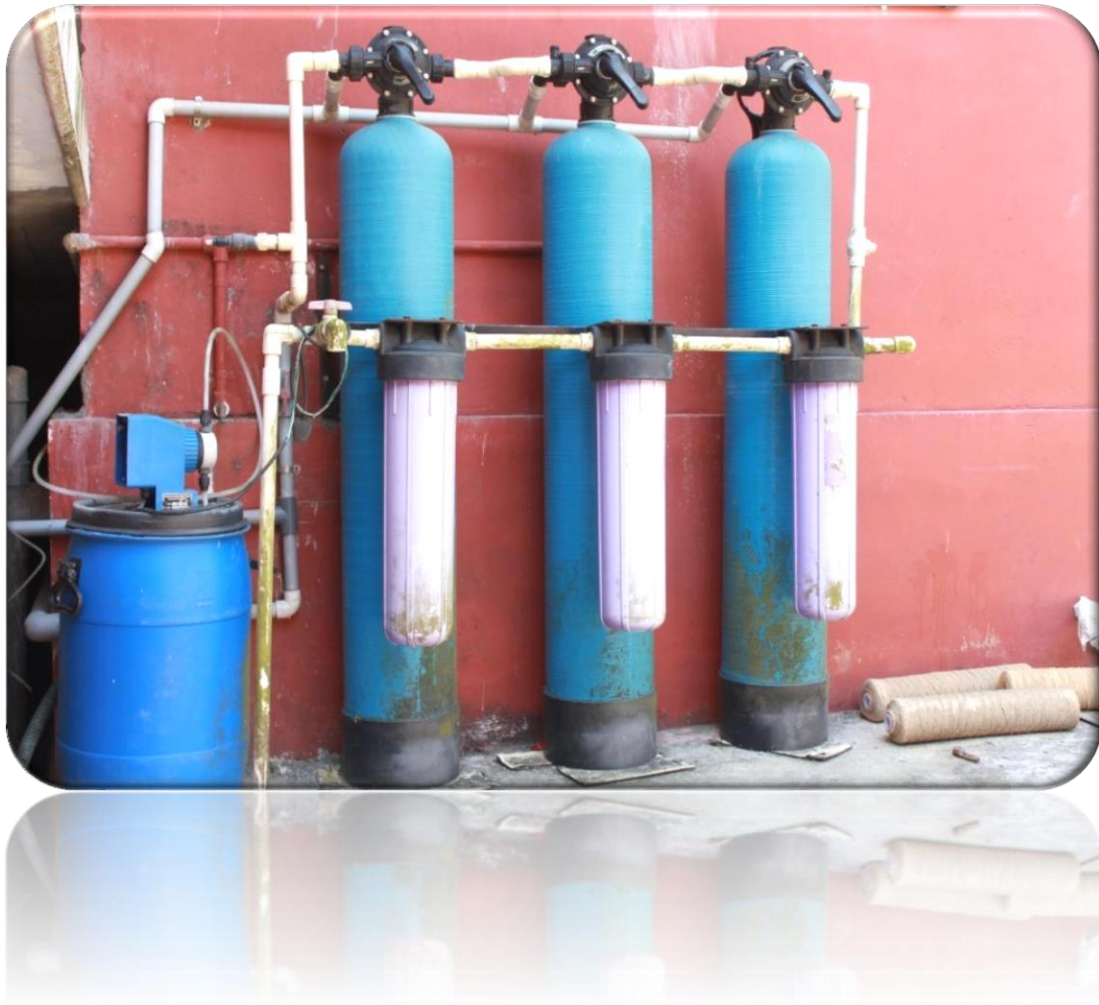
Water purification units
