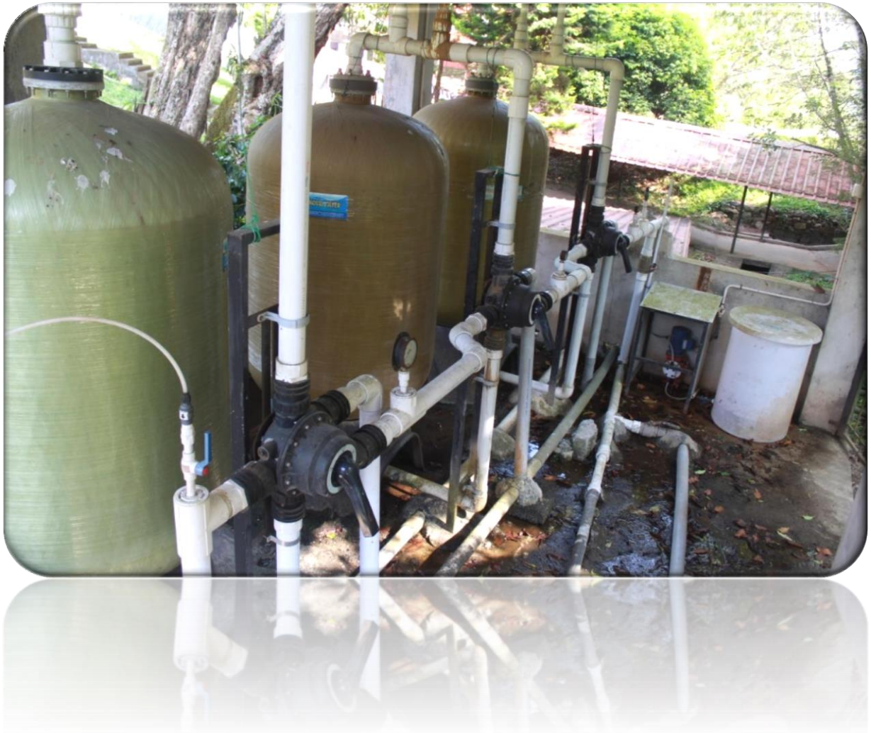
Water filtration systems
