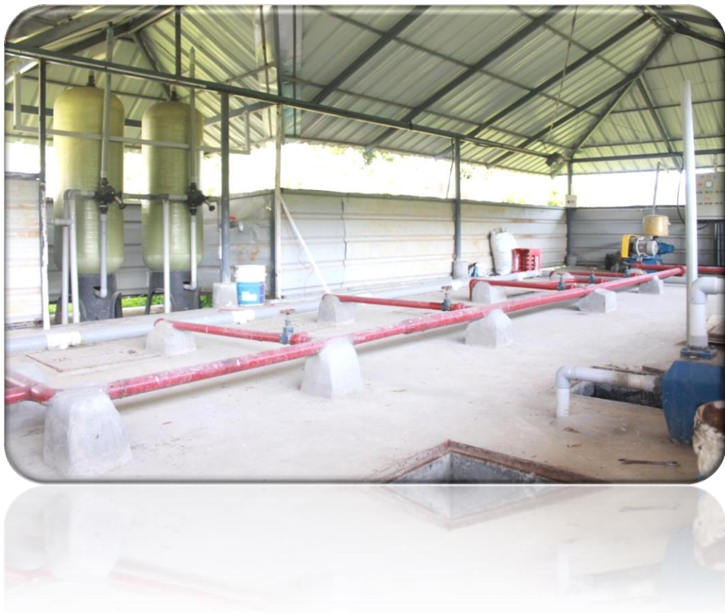
Sewage Treatment Plant with a capacity of 50,000 litres/ day
